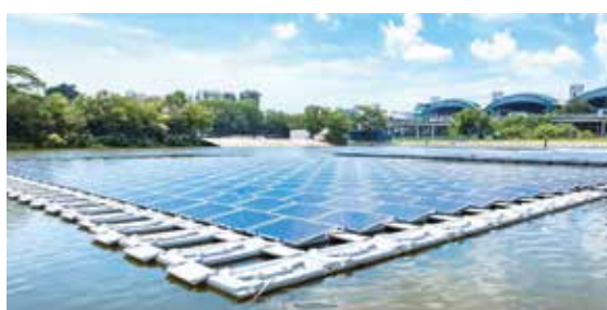
Floating PV installations
